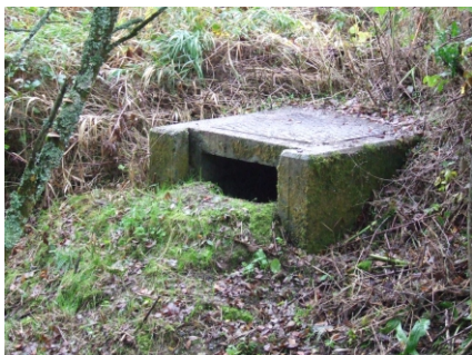
Entry pipe to filter bed
